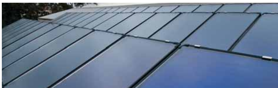
BT collectors at Rheem Testing Facility – Rydalmere – Australia
